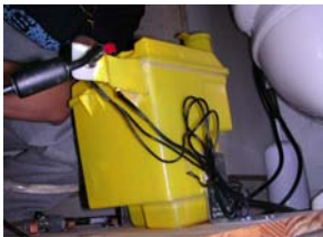
Figure 12.11. One-Gallon Soap Tank
