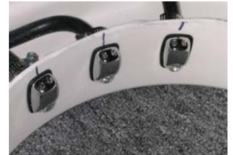
Figure 12.7. Water Spray Nozzles
